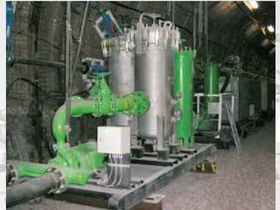
Stationary pump station for HFA supply
