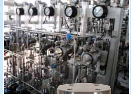
Chemical Injection Skid
