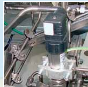
Pressure Transducers on compressors to monitor different pressure stages.
