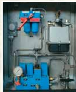
Change-over-filters in pipeline shut-off valve control unit.
