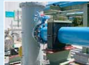
Mounting of pipes on oil rig with HYDAC Clamps and RFL Filter with offshore coating.
