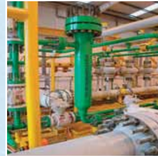
Mono Ethylene Glycol (MEG), Filter, used for gas dehydration on offshore platforms
