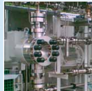
Methanol compressors using Stainless Steel Filters - HPSSF. 10,000 psi (690 bar)
