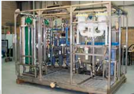
Filters, Ball Valves, and Accumulators in HPU unit.
