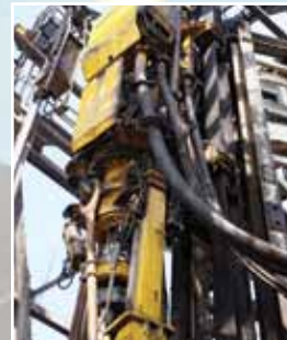
Drilling Top Drive powered and controlled by HPU and controlled by valve block.
