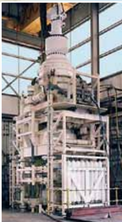
Accumulator Station in BOP
