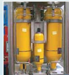
High Pressure Accumulators , providing sufficient capacity to operate 100% of all the valves on a production tree.
