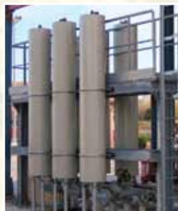
Piston Accumulators used as surge alleviators on truck loading terminal.
